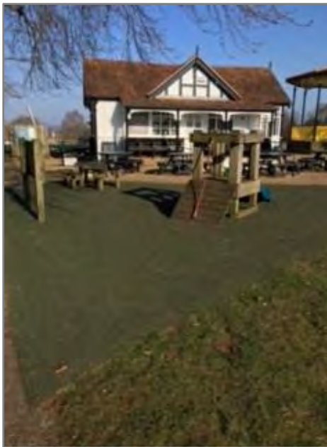
A new safety surface was installed in the play area in Vine Gardens .
