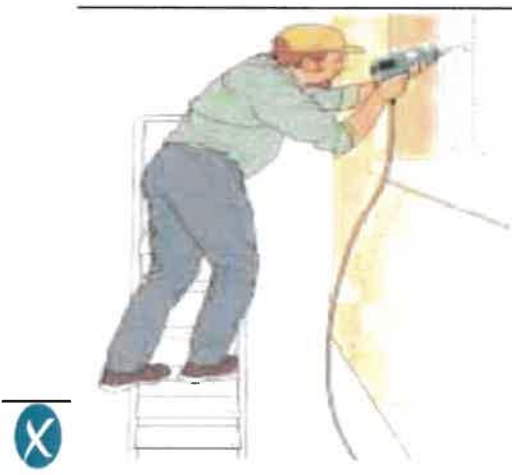
Incorrect – steps side on to work activity
