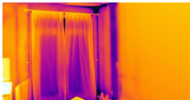
Darker areas around doors and windows show draughts.
